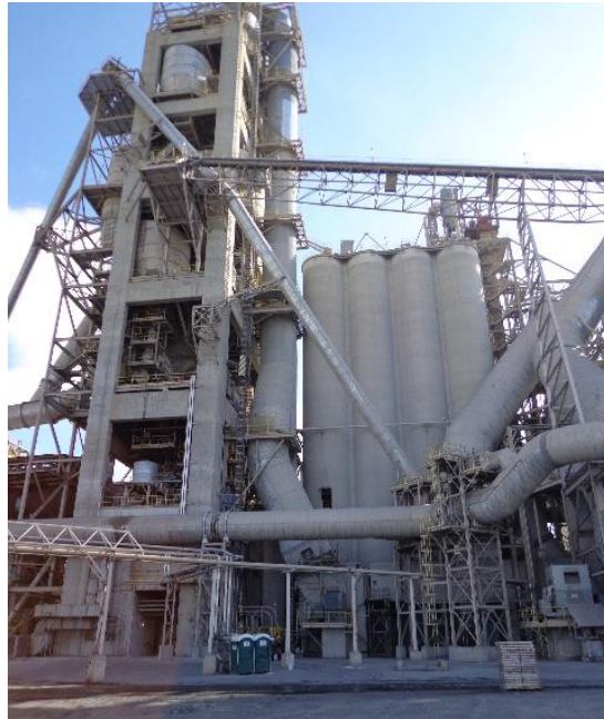
Fig. 1. High temperature fan technology was installed for the main Kiln ID fan at the South Carolina plant.
