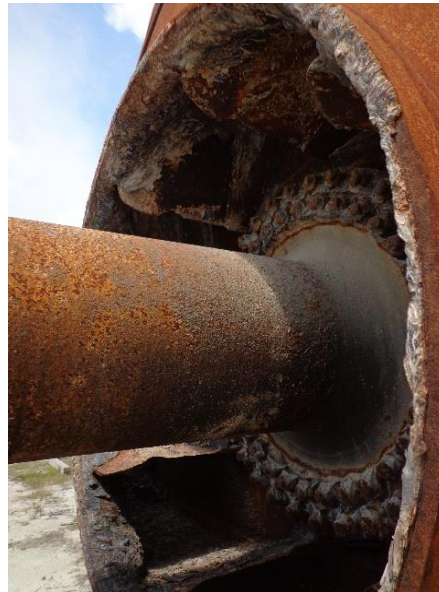
Fig. 2. Thick hard build up and wear on the old fan surfaces, requiring frequent maintenance.
